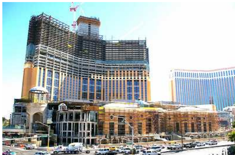
New casino in Las Vegas called "Palazzo" containing approximately 70,000t of structural steel. Detailed by BDS Steel Detailers – Brisbane
